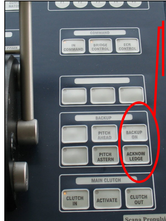
ME CPP control at Fore Bridge
